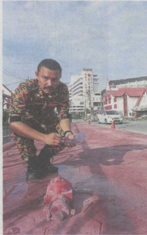
South Klang Fire and Rescue Department officer Mohd Faizal Samsudin taking note of the fire hydrant that is covered with concrete along Jalan Mohet in Little India.
